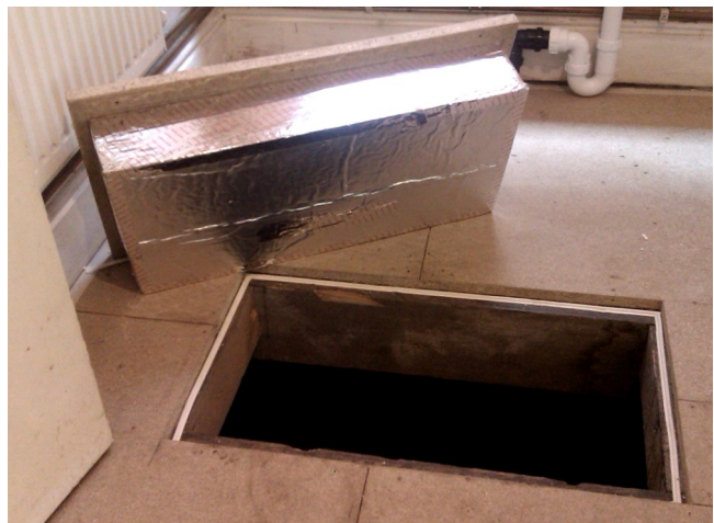
Floor hatch showing draught strip around the lip. For an attic hatch the insulation would be on the topside.
