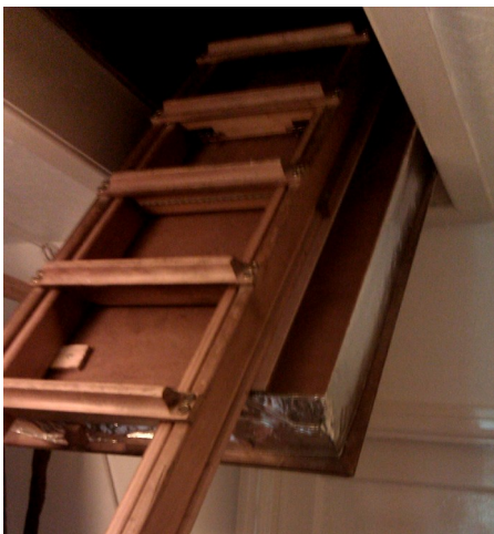
Insulated attic hatch above a ladder
